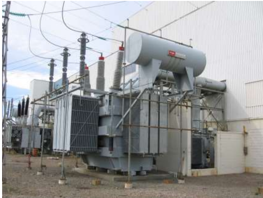
Figure 1: Holyrood T2 Transformer
