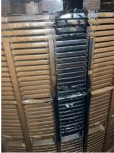
Figure 2: Holyrood Transformer T2 Failed High Voltage Winding
